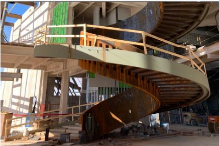
Buddy Holly Stairs - Developed custom connections and custom erection aids needed to safely fabricate and install the stair. Construction Engineering
